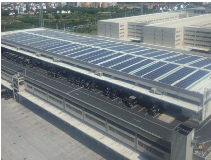
Photovoltaic power station at Yiwu Industrial Park
