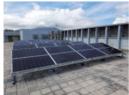
Photovoltaic power station at Hong Kong Industrial Park
