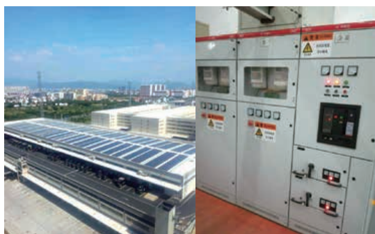
Photovoltaic power station in Yiwu industrial park
